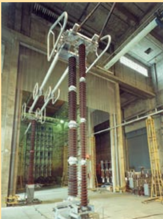
OH 550 kV 6300 A
