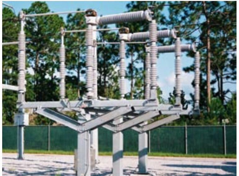
CSH-B 242 kV replacing DS+CB on a single structure
