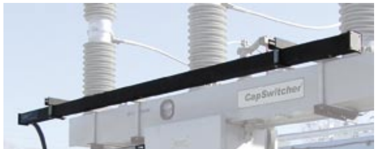
CMD® sensor installed on a CapSwitcher®
