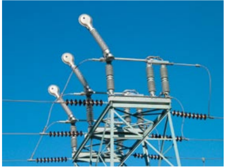
VSD 123 kV installed to sectionalize a line
