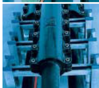
All fixed. Anchoring clamps for fixing cables against longitudinal stretching in steep terrain.
