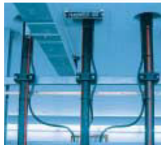
Fastening in basement. Alignment and fastening of high-voltage single-core cables in cable basement.
