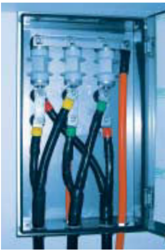
Cross-bonding link box. For the cross-bonding of cable screens. The surge voltage arrestors protect the outer sheath of the cable from both switching and atmospheric over-voltages.
