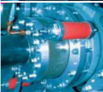
Safely protected. Sheath overvoltage arrestors across the isolated part of the SF6 sealing end protect the outer sheath from surge voltages.
