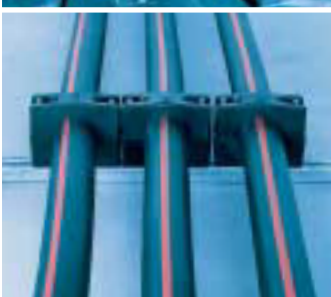
Good routing. Synthetic rubber clamps for fastening and alignment of cables to required route.
