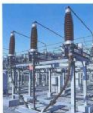
Open Air. Outdoor plant in operation.
