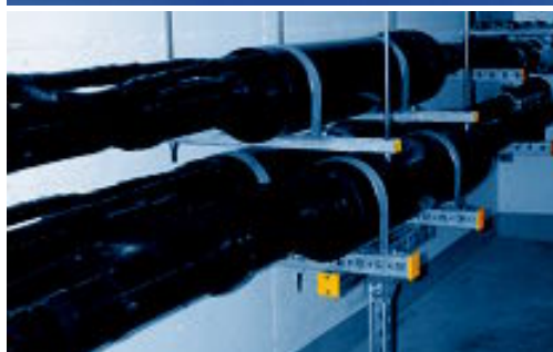
Laying in a tunnel. Joints with Cu-tube and HDPE-coating in a tunnel.
