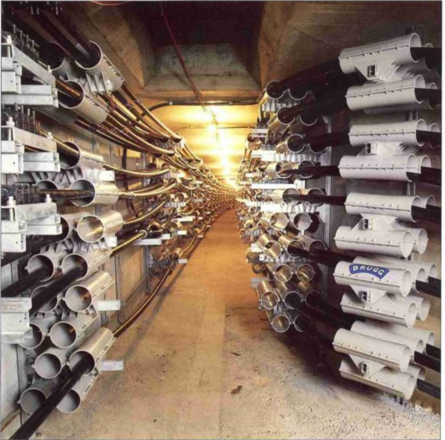
EWZ, Cable tunnel under Löwenstrasse, Zurich (Switzerland)
